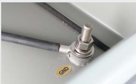
Internal ground stud to accommodate factory provided neutral terminal ground wire and incoming cable grounds and shields.
