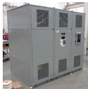
Medium Voltage Ventilated Substations
