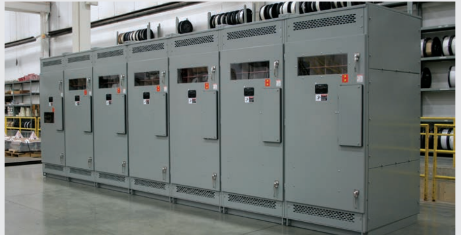
Load Interrupter Switch
